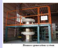
Biomass generation system
